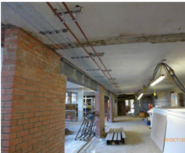
Exhibition Space: General View (NB: Work in Progress: new openings formed to increase foot print & installation of service pipework).
