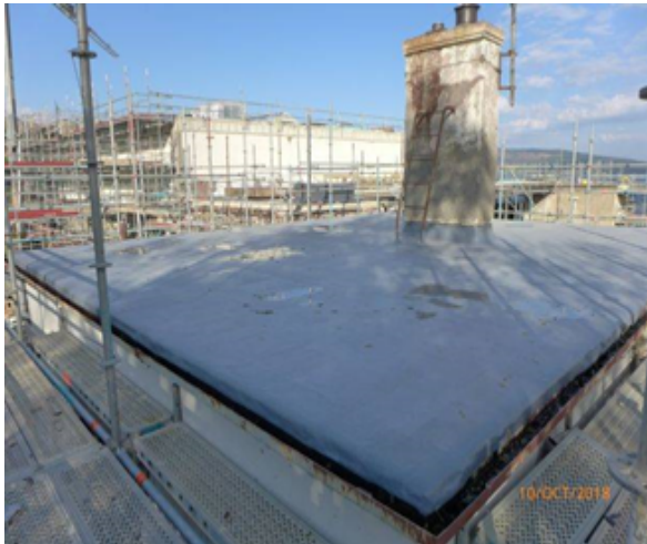
Looking North: Caretakers House Roof (NB: Fly Tower south elevation visible in background).
