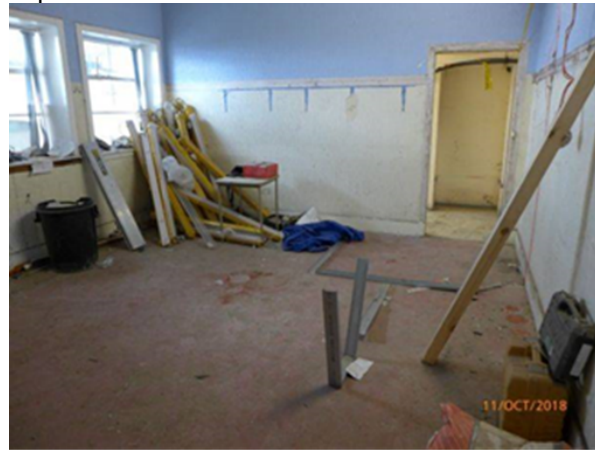
Green & Communication Rooms: (NB: Work in Progress - bottom track installation for creation of new partition walls).
