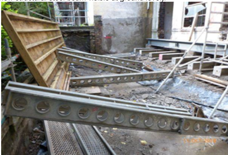
Shop Area: Work in Progress to create new extension to increase Shop floor area.
