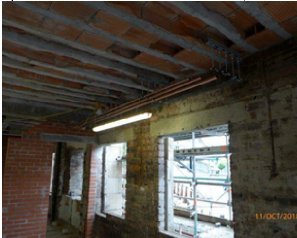
Back Stage: Changing/WC Area: General View (NB: Work in Progress: new dividing walls visible including installation of service pipework).
