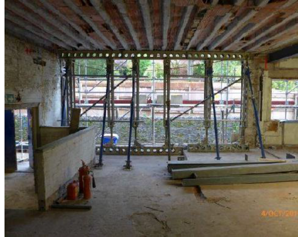
Stage loading bay Area (Adj. Stage Area) (West/Rear elevation): enlarged opening to improve access.
