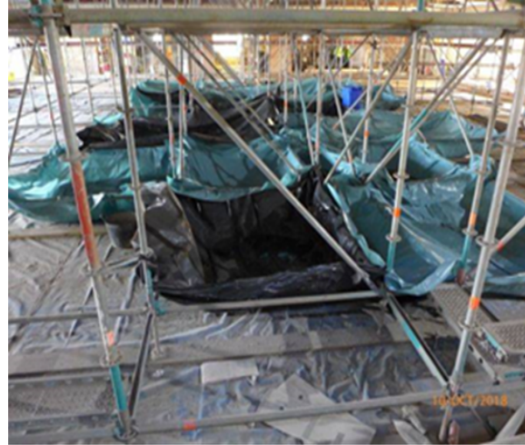
Auditorium/Main Hall: (NB: additional rainwater protection in situ below main roof light) – lack of over roof is proving challenging due to adverse weather conditions.
